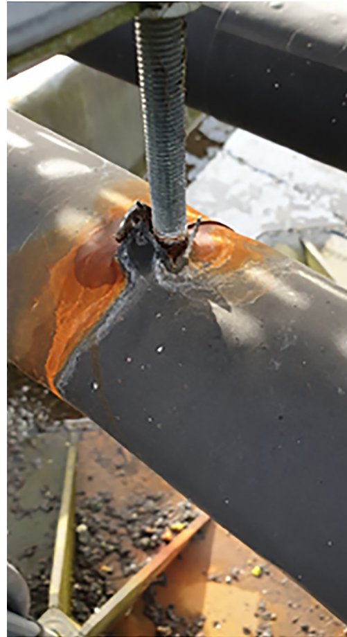
Fig. 4 Bracket penetrating weatherproofing leading to corrosion
