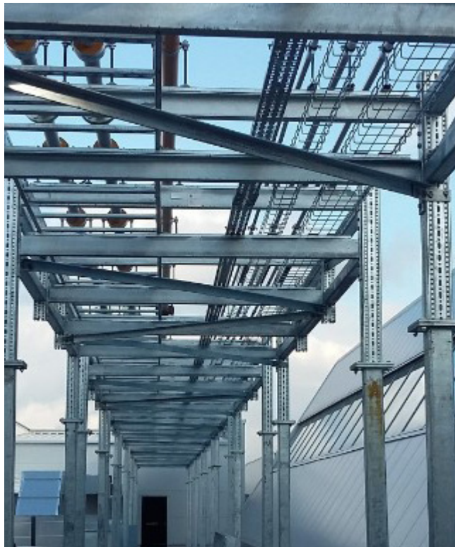
Fig. 1 Multi services gantry on external plant deck.
