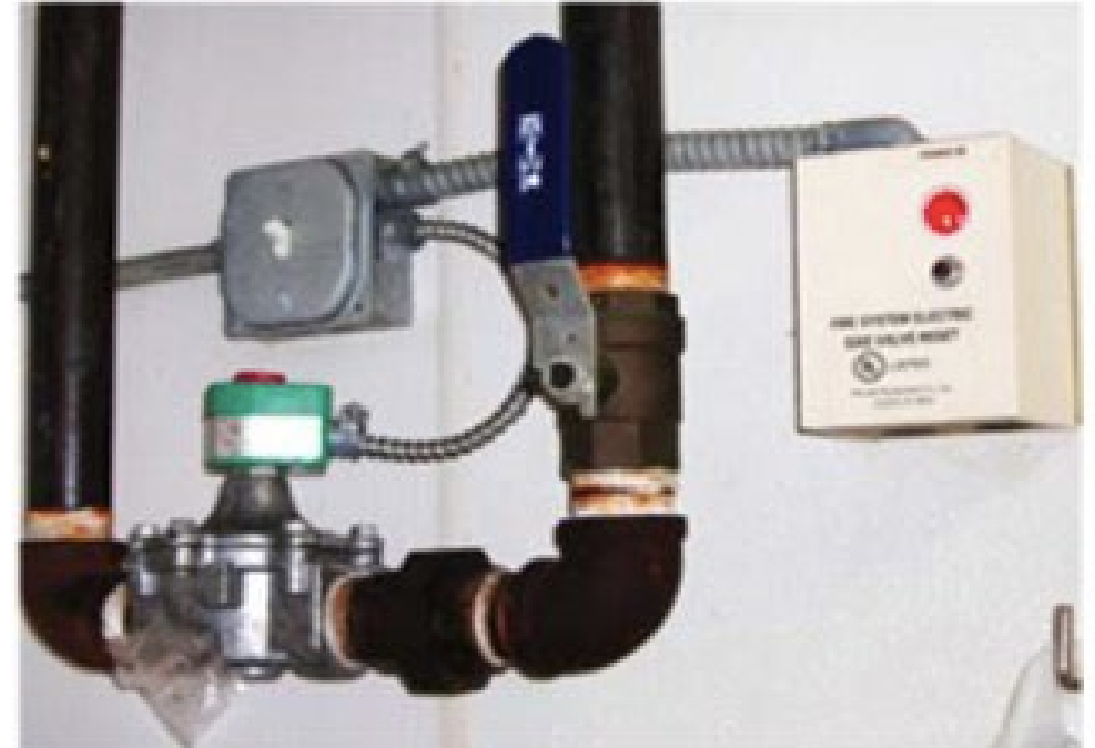
Example of automatic gas isolation valve
