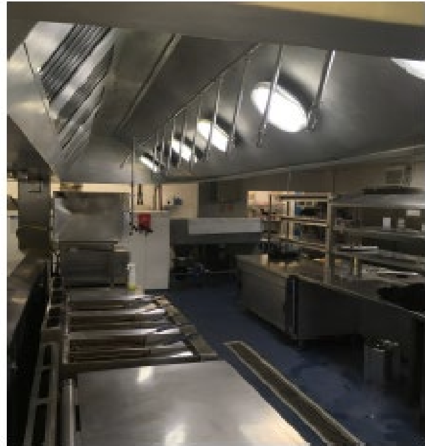
A Photograph of a Kitchen Fire Suppression System
