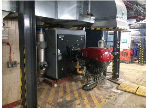
Replacement boiler plant installed in 2017
