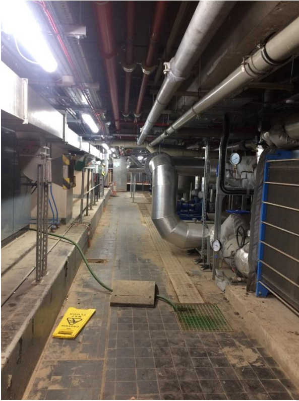
Plant rooms contain asbestos both in the containment lining and fabric of the structure
